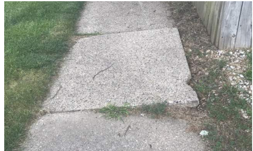
Figure 4.5: Heaved Sidewalk Panel
