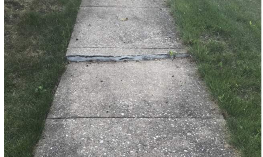
Figure 4.4: Cracked and Sunken Sidewalk Panel
