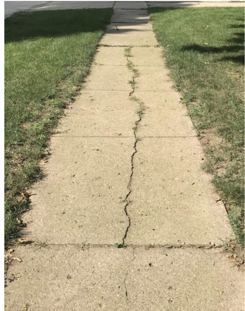
Figure 4.6: Cracked Sidewalk Panels
